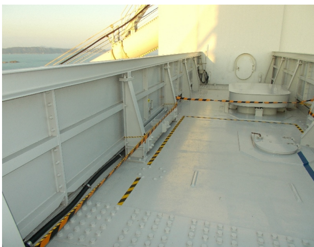
Watch Your Step Protruding Bolts
